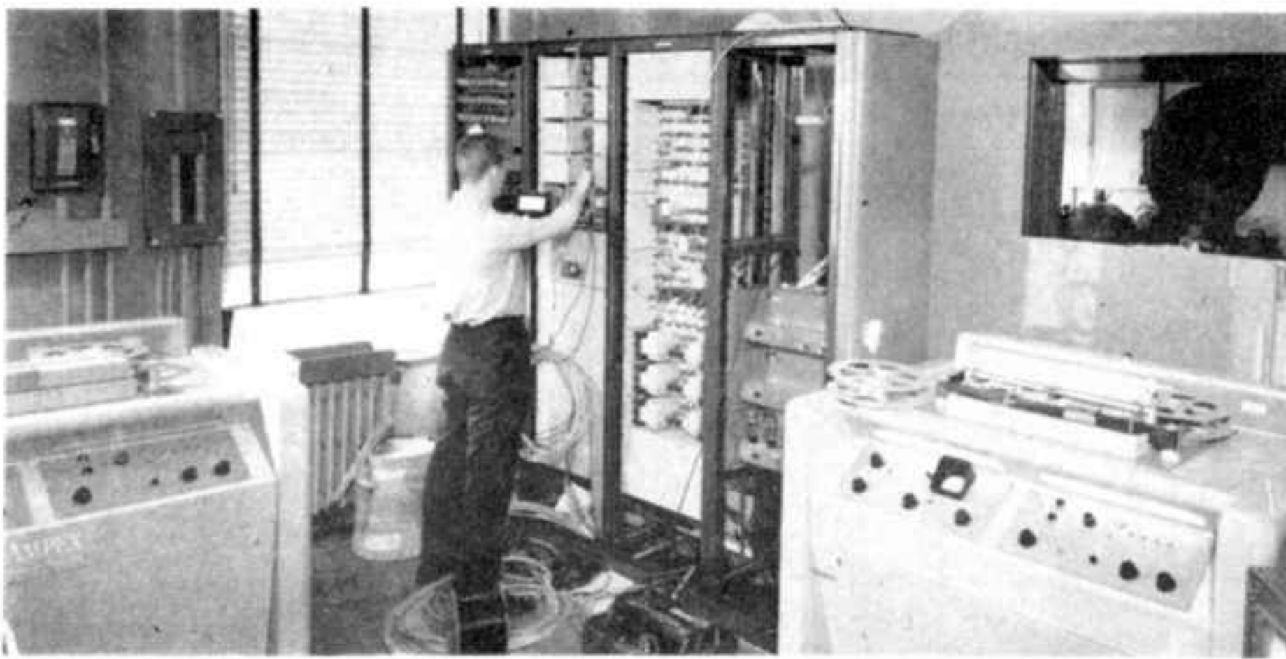
Technician wires rack equipment in ABC's Chicago video-tape recorder installation
